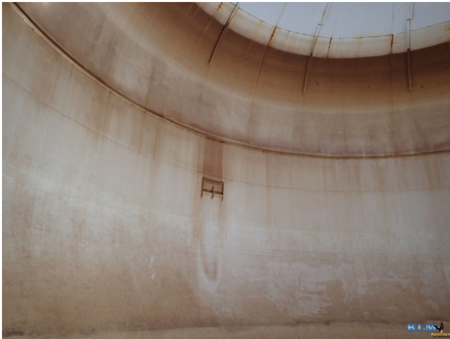
Photo No. 8 Shell coating conditions
