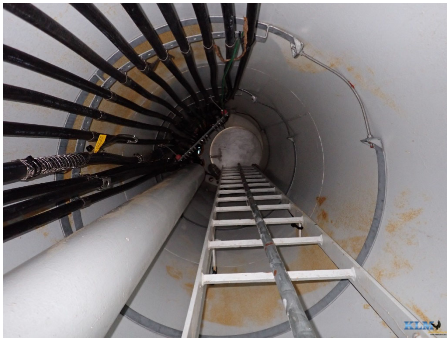
Photo No. 36 Coating failures visible in drywell tube
