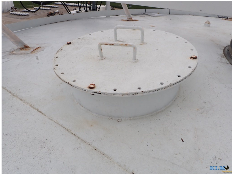
Photo No. 61 Ventilation manway on roof
