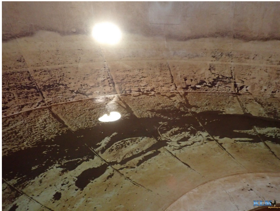
Photo No. 12 Bowl conditions prior to cleanout
