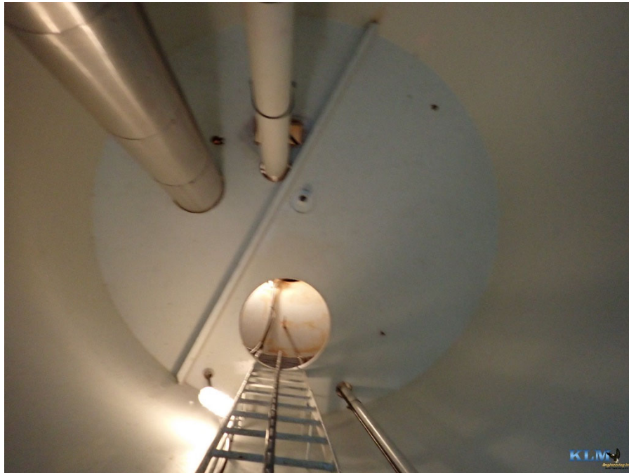
Photo No. 47 Underside of top landing conditions
