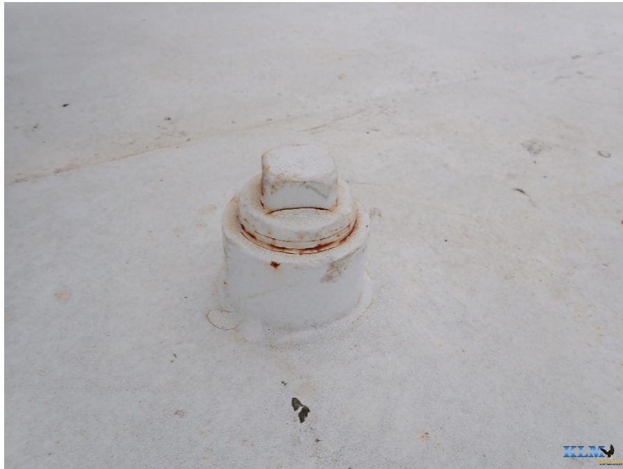
Photo No. 59 Roof rigging coupling
