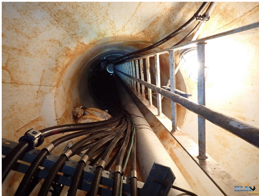
Photo No. 40 Bowl coating conditions
