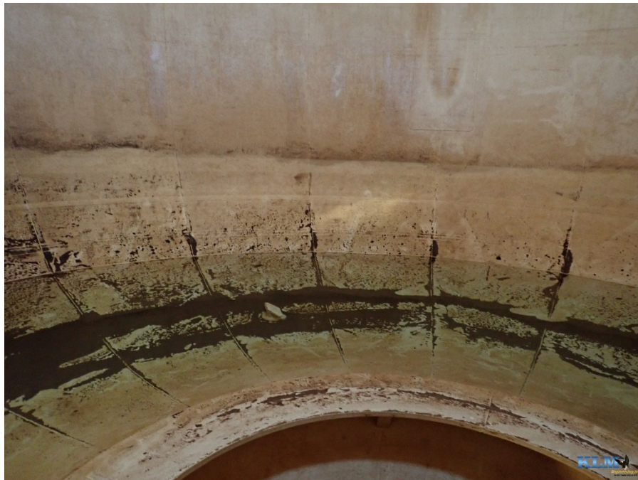
Photo No. 14 Bowl conditions prior to cleanout
