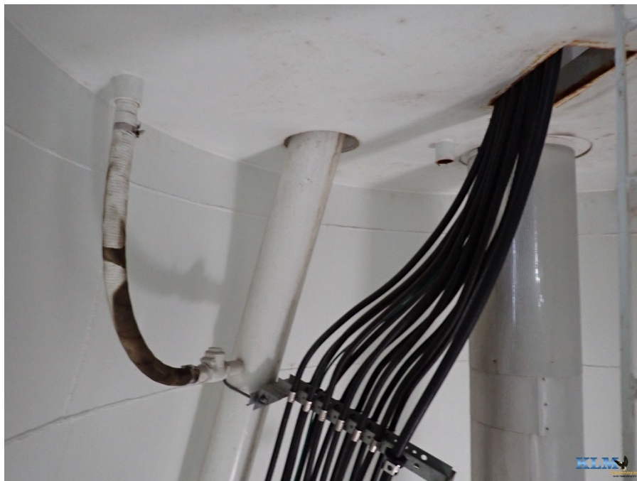
Photo No. 50 Underside of bottom landing with overflow pipe and fill pipe penetrations
