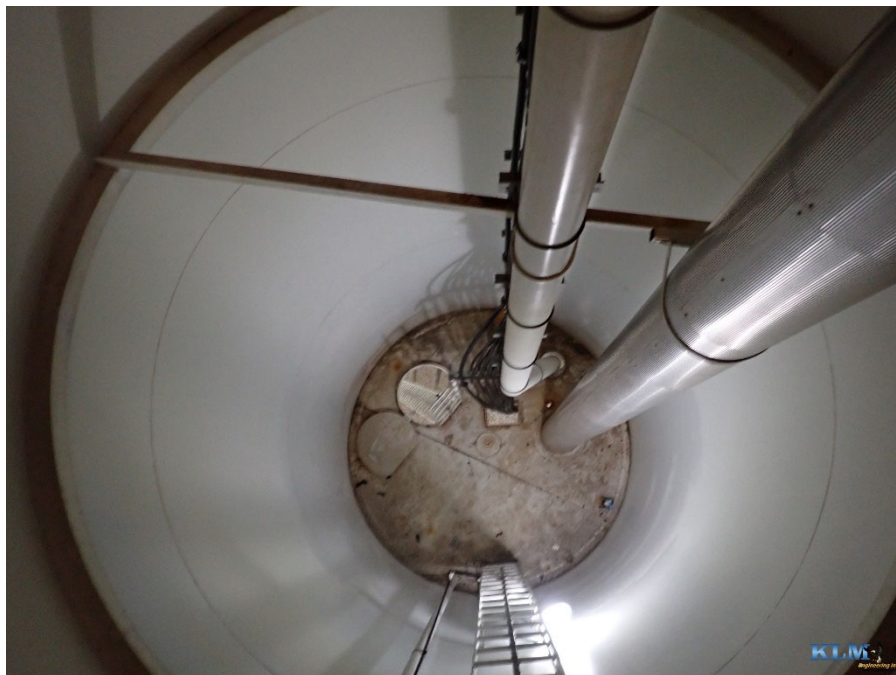
Photo No. 48 Pedestal conditions looking down at bottom landing
