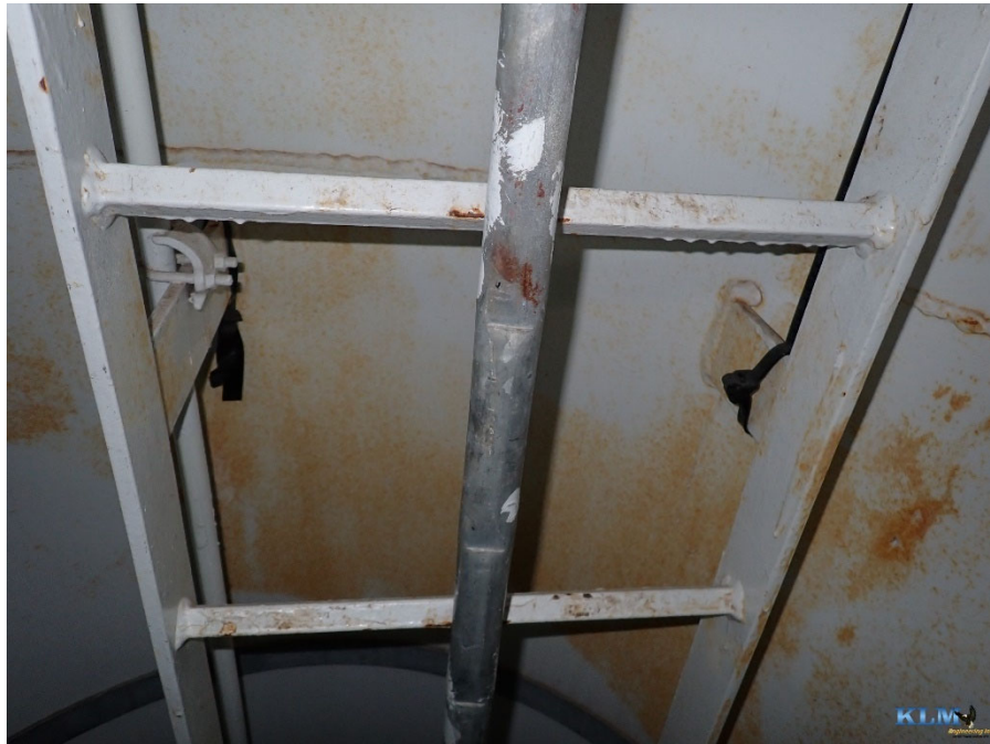
Photo No. 37 Drywell tube interior conditions
