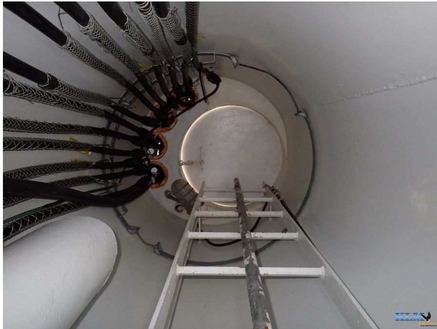
Photo No. 35 Coating conditions of drywell tube interior
