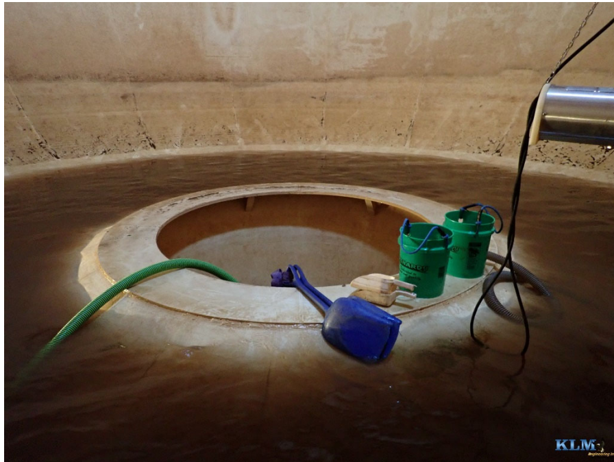
Photo No. 15 Bowl conditions prior to cleanout
