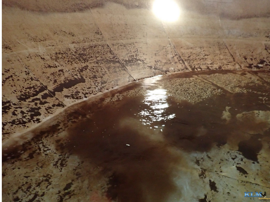
Photo No. 13 Bowl conditions prior to cleanout
