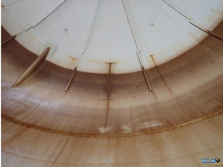
Photo No. 7 Upper torus and shell conditions
