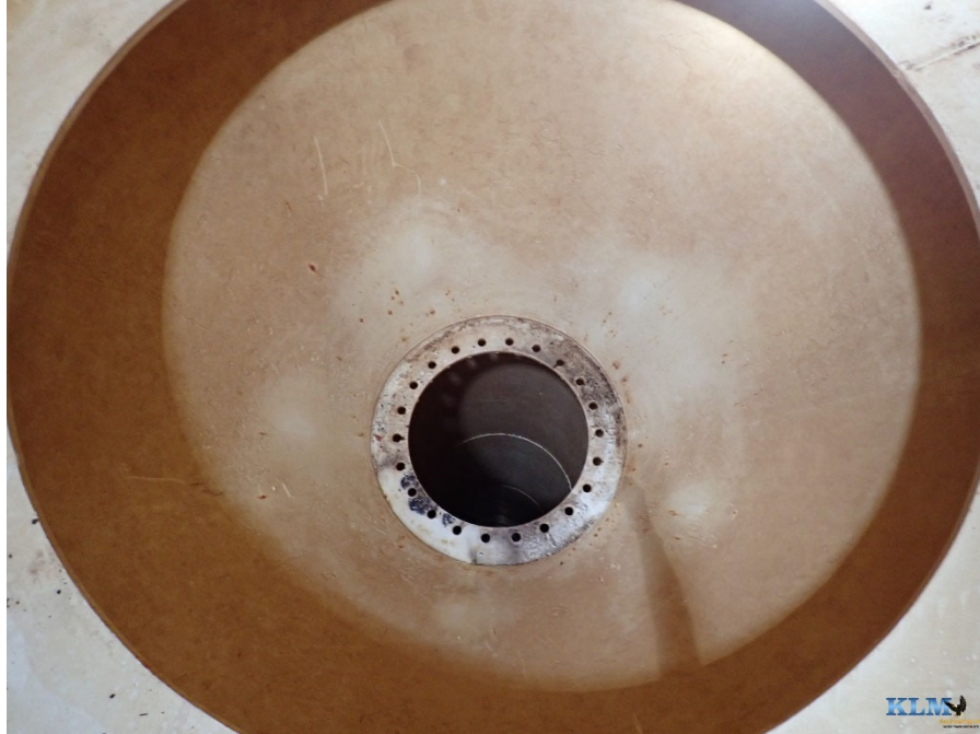
Photo No. 19 Cone and top of wet riser
