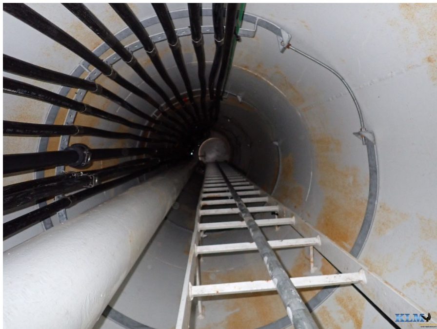
Photo No. 38 Drywell tube interior conditions
