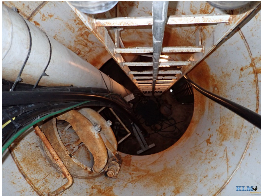
Photo No. 39 Coating failures within base of drywell tube
