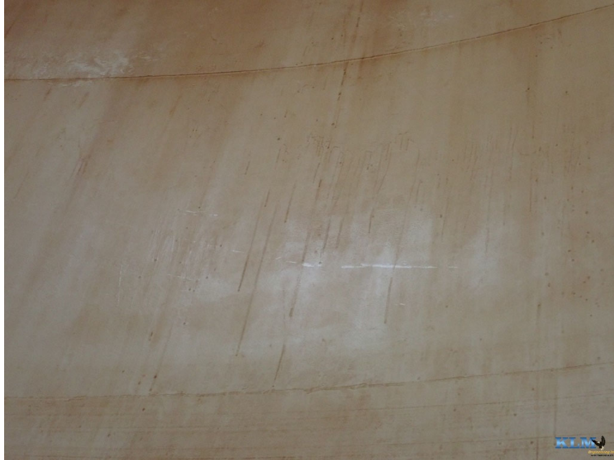
Photo No. 11 Shell coating conditions
