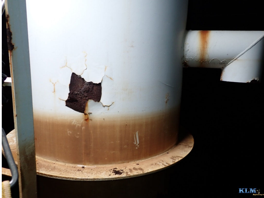
Photo No. 15 Drywell tube with overflow pipe inlet visible Advanced corrosion visible
