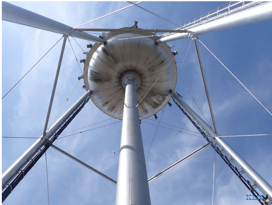
Photo No. 40 View of wet riser and columns
