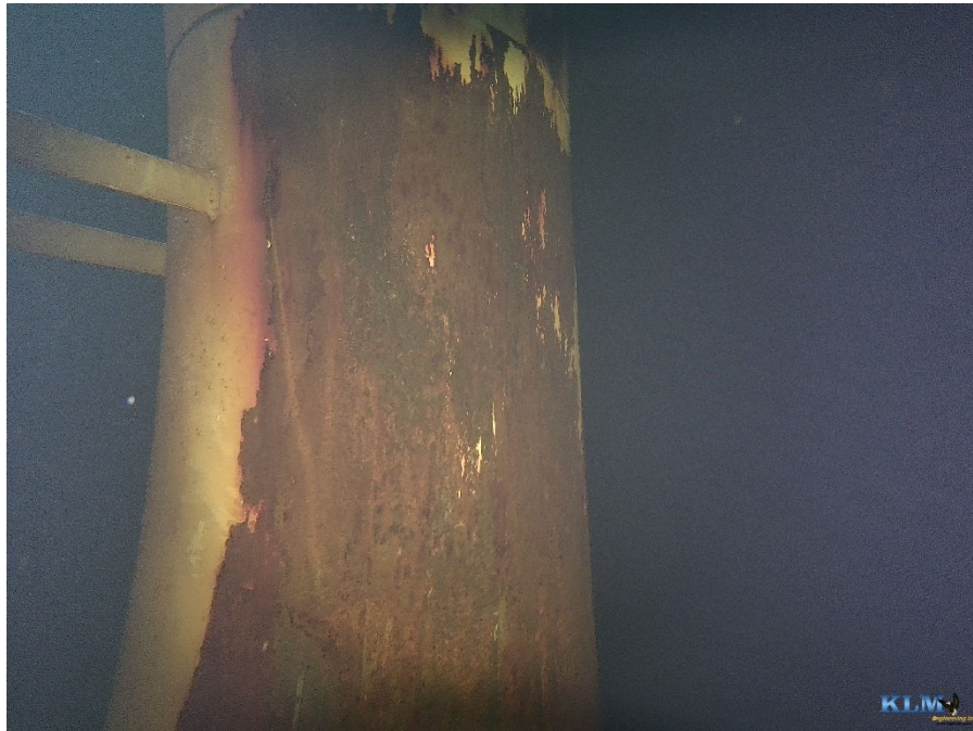
Photo No. 19 Conditions of coating failure on drywell tube
