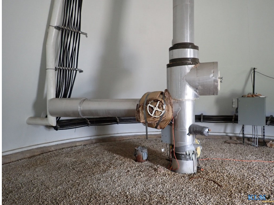
Photo No. 53 Conditions of base cone with fill pipe and overflow pipe
