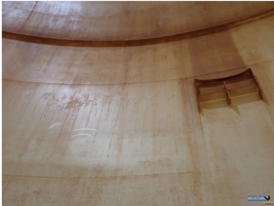
Photo No. 9 Shell coating conditions
